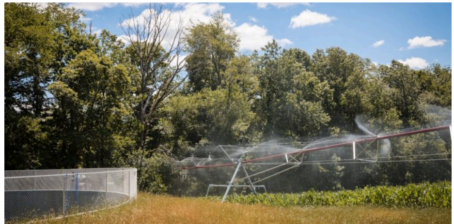
The Jellystone Park Quarryville has unveiled an innovative wastewater solution that benefits a local farmer. Credit: Jellystone Park Quarryville
